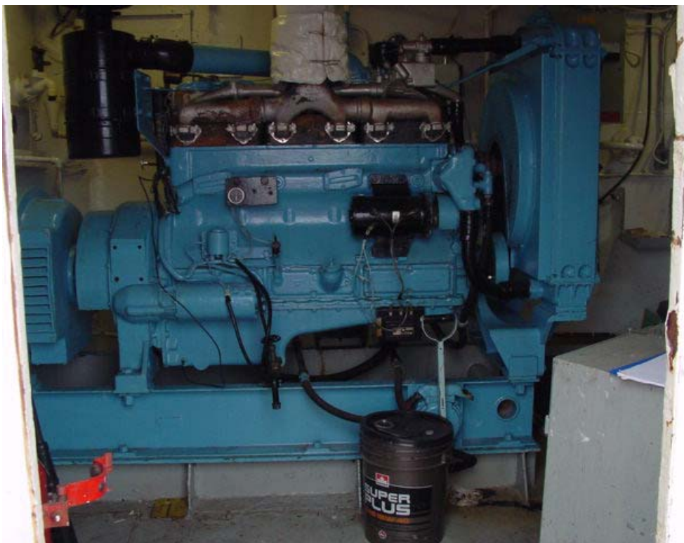
Photograph 2: General view looking at the Emergency Generator.
