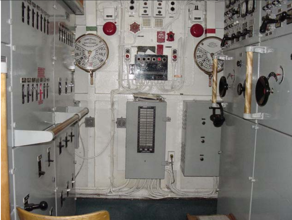
Photograph 4: View looking aft in the Control Room between the switch boards.
