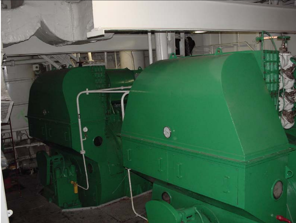
Photograph 5: General view looking aft to starboard in the Propulsion Motor Room.
